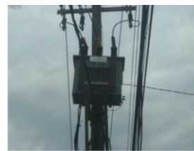
Gambar 4. Trafo Distribusi Step Down
