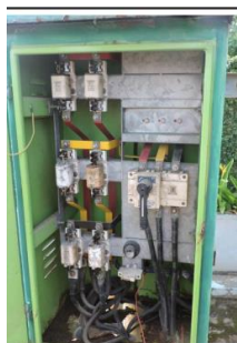
Gambar 3. Box Panel PHB TR
