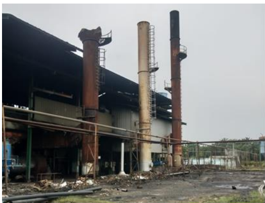
Figure 1. Infrastructure Corrosion on Industry of PTPN 1 Cot Girek (by research).
