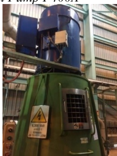
Gambar 5. Hot Well Pump P400A di PLTP PGE Kamojang Unit IV
