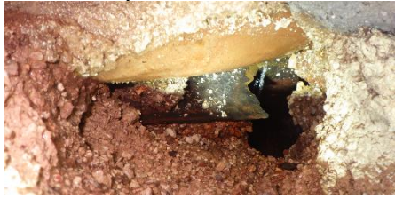
Gambar 5. Kebocoran Pipa Boiler
