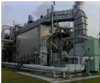
Gambar 3. Boiler Kilang Pertamina [5]
