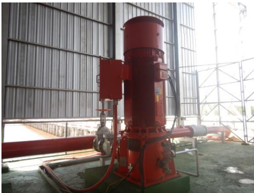
Gambar 1. Fire Pump 717-P-3
