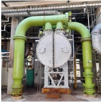
Gambar 4. CO 2 Compressor surface condenser (D2-302-JTC-K2)
