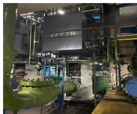
Gambar 2. Motor Condensate Extraction Pump 10,5kV
